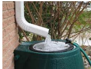
Rain barrels capture stormwater for re-use
